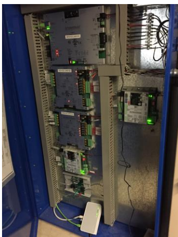
DDC panel boiler room
