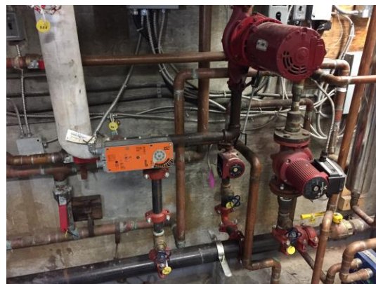
Heating Circulation Pumps
