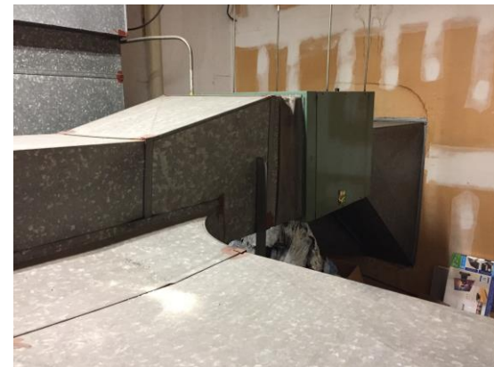
Gym Changeroom Exhaust Fan
