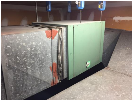
Pool Changeroom Exhaust Fan
