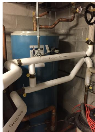
DHW Storage Tank
