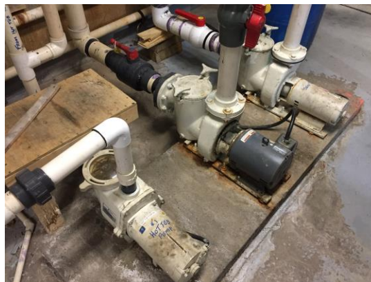
Pool Circulation Pumps
