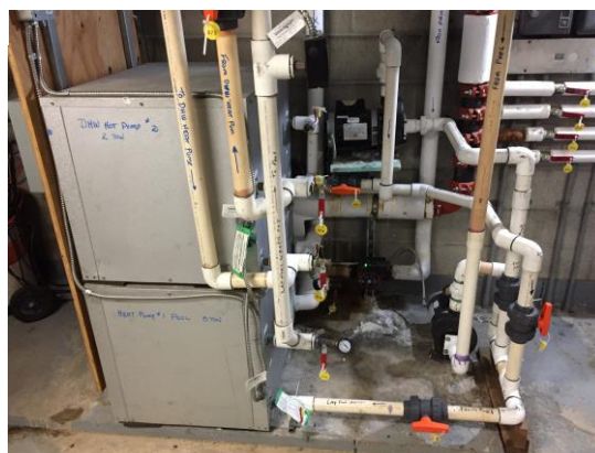
Heat Pumps & Circulation Pump
