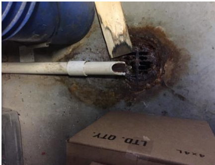
Rotted floor drain
