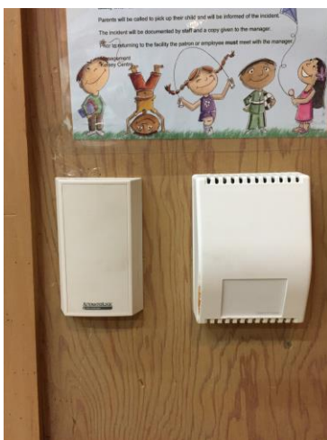
DDC temperature sensor
