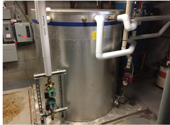
Solar Drain Down Tank
