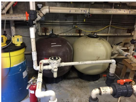
Pool Sand Filters
