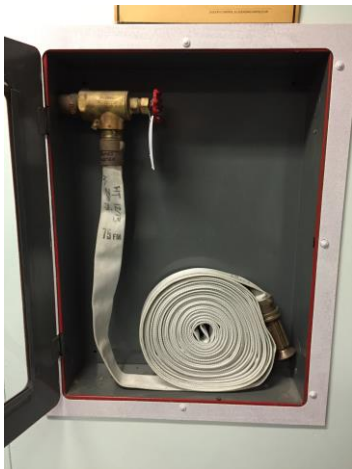
Fire Hose Cabinet
