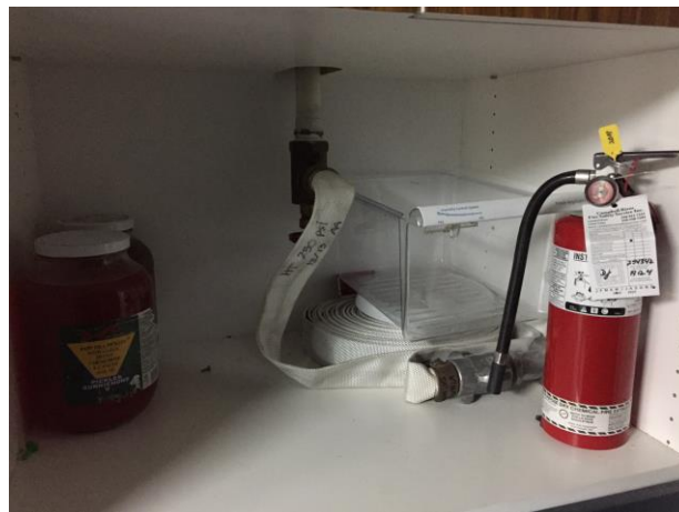
Fire Hose & Extinguisher
