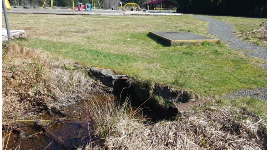
Photo 9 - 600mm CSP pipe inlet to DMH 2
