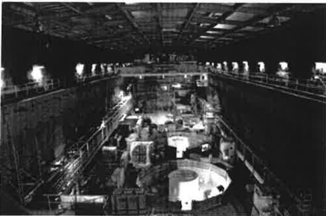
A July 2018 view from the service tunnel into the powerhouse cavern. Two of the three turbines/generators are the circular works.
