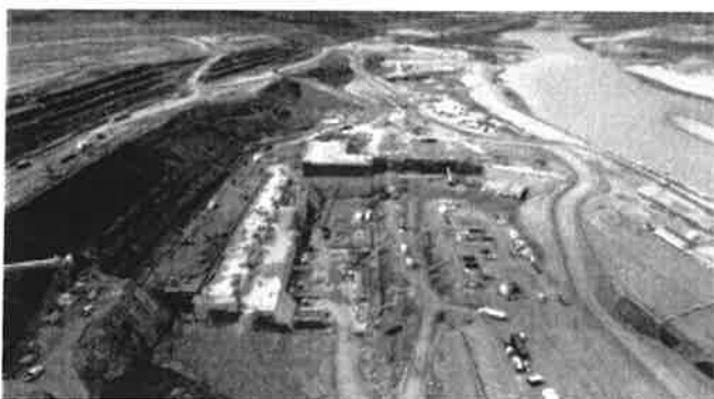
The Site C powerhouse buttress and main service bay pad, looking upstream, in August 2018.
